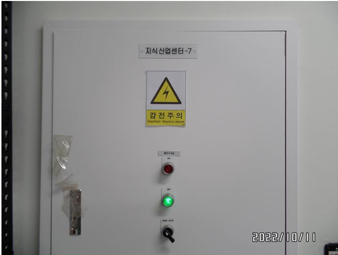
Electrical control panel
